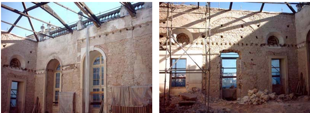
Fig. 6.16 – Restoration works at the 18 th century Laboratorio Chimico, University of Coimbra in February 2005. The Laboratorio also includes an amphitheatre. During restoration, a couple of 16 th century architectural elements (window and pulpit, not depicted) were discovered (reproduced with the kind permission of the University of Coimbra).
