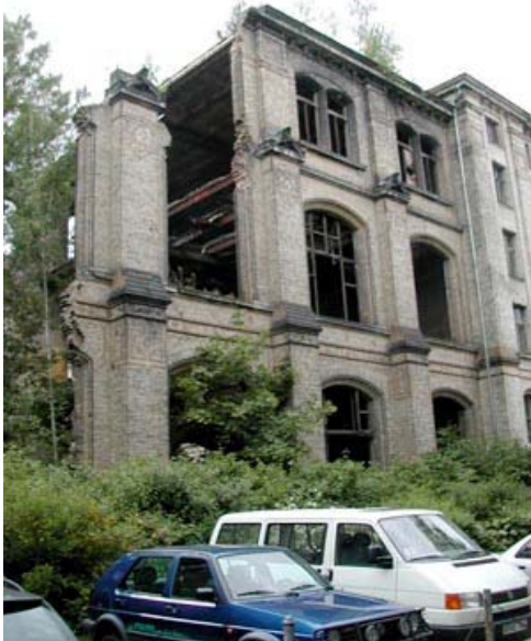
Fig. 5.13 - Museum of Natural History, Humboldt University Berlin, damaged by World War II bombings. Photo taken in July 2004.
